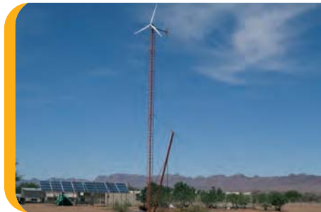
Betta Campsite's hybrid power system [Source: THI]
